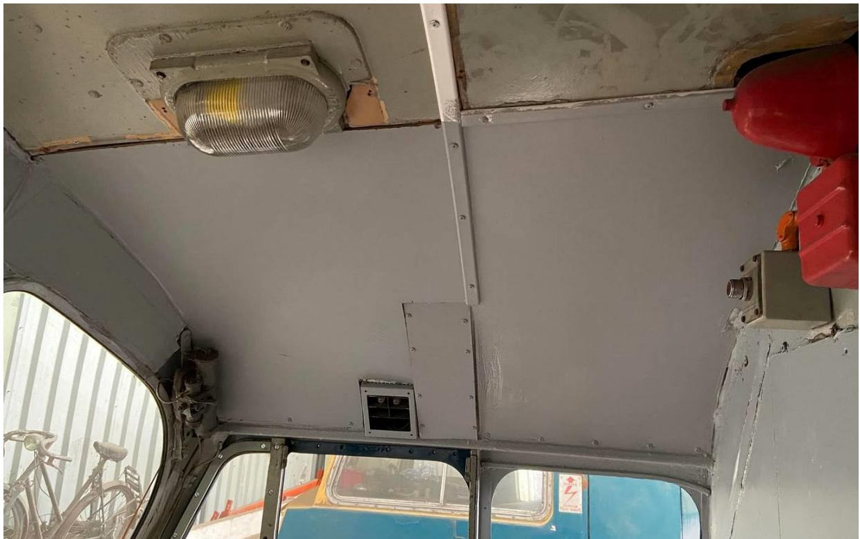
Gloss paint being applied to the new ceiling panels in No.1 cab. 07/08/22
